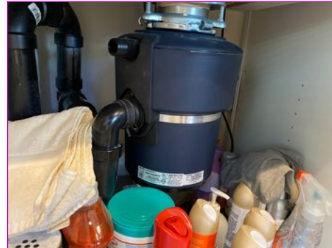
Plumbing under sink 2
