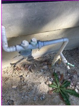
Water lines at the home.
