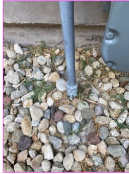
Main shut off
