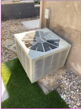
Air conditioner condition
