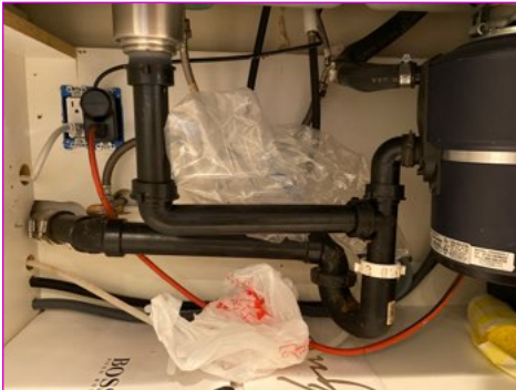
Plumbing under sink
