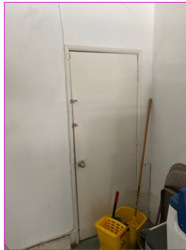
Garage exterior door is visible out of square
