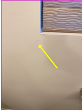
Corner cracking noted at window
