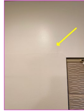
Corner cracking noted at window
