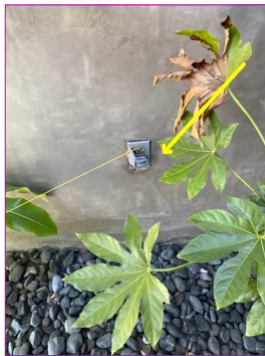
Electrical outlet at the front left of entry way not functioning.
