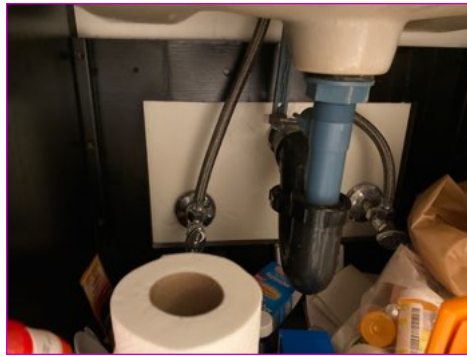
Plumbing under sink
