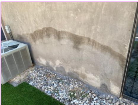
Stucco damaged at the rear left wall.
