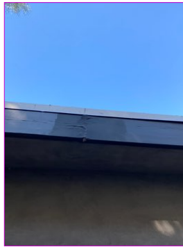
Moisture damage noted at right side fascia boards
