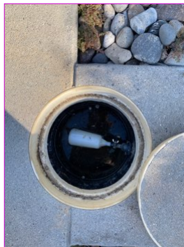
Auto fill device did not function properly at the time of inspection.
