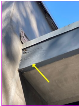
Moisture damage noted at front fascia boards.
