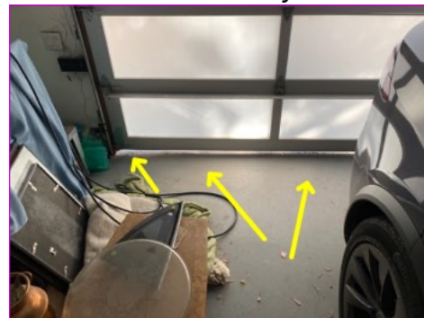
Garage door does not seal at the base when closed.
