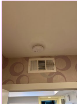
Smoke alarm in place and functioning
