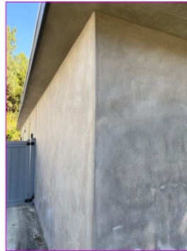
Cracks in exterior wall
