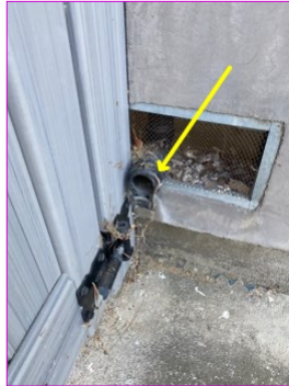
Plumbing drain cap damaged/missing at the left side of home.
