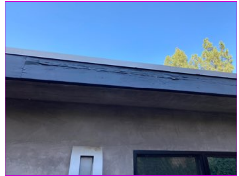
Moisture damage noted at the right side fascia boards
