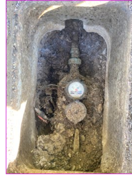
Main water line
