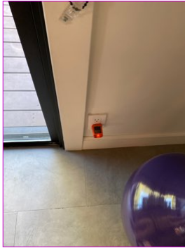
Electrical outlet on the rear wall of living area near the sliding glass door wired with open ground wiring.
