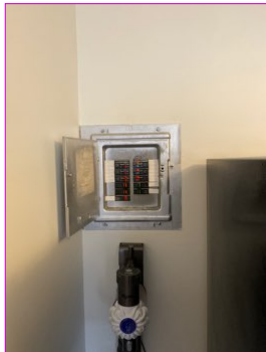
Laundry sub panel
