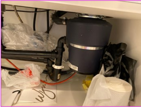
Disposal under kitchen sink was not functioning at the time of inspection.
