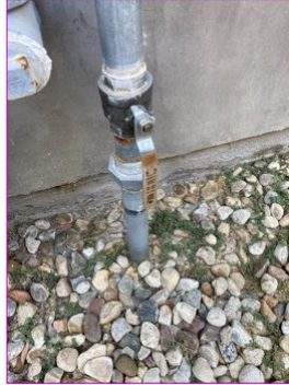
Shut off valve
