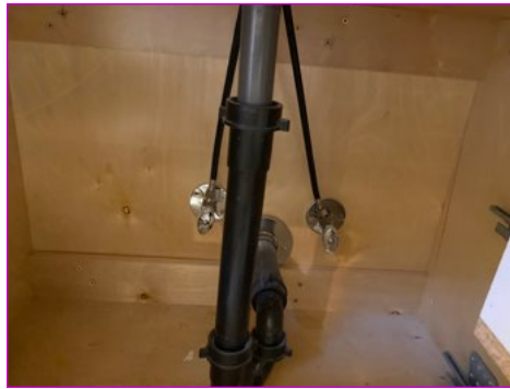
Plumbing under sink
