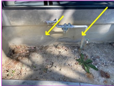
Cracks and deterioration noted at the front foundation large coat.
