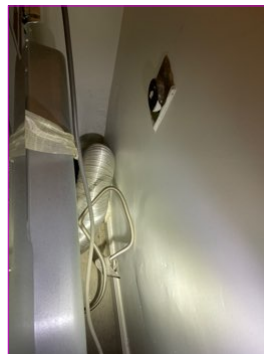
Gas and vent pipe
